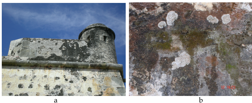
Fig. 11. Aspect of the biodeterioration in the historic buildings of San Francisco de Campeche City. (a) Fort San Carlos. (b). Microbial community at West wall of Fort San Pedro.
