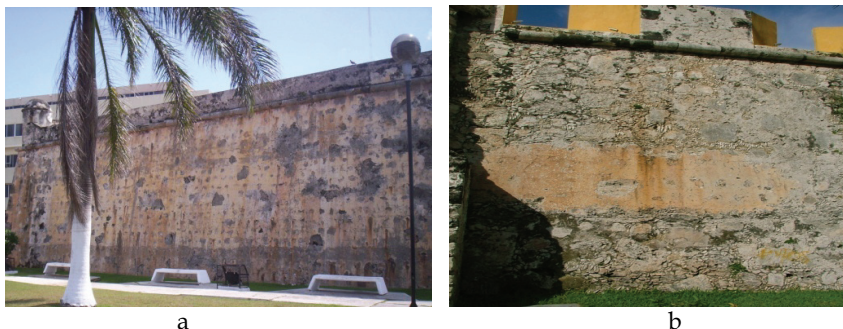
Fig. 2. General aspect of degradation at Forts San Pedro (a) and San Carlos (b), historic buildings of San Francisco de Campeche City.
